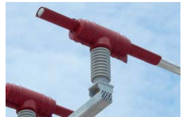
2 MVLC-38 on busbar with BCIC
