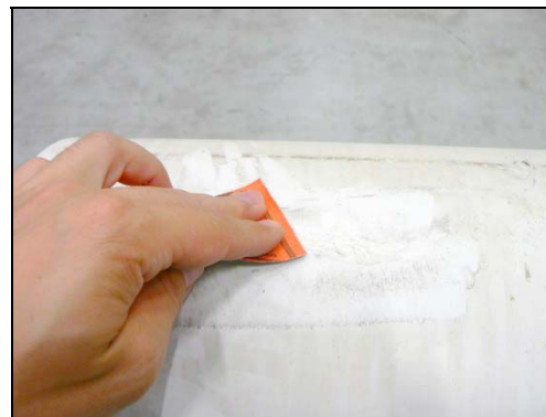
The applied repair material can be smoothed with a spatula. Remove any protruding material with sand paper, scraper or grinding tool to achieve a flush finish with the PP line coating.
