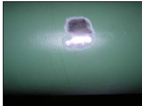
Damage in FBE line coating > 10 cm 2
