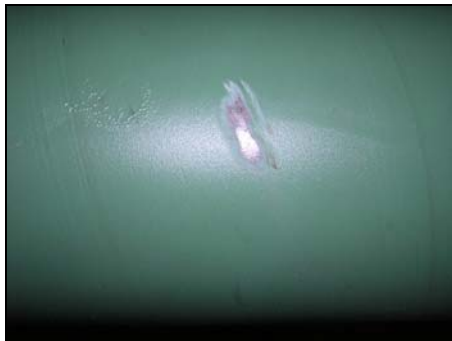
Scratch in FBE line coating.
